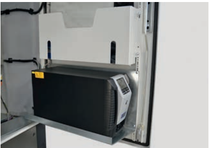
Uninterrupted power supply Safeguarding of the control computer and controlled shutdown in case of power failure.
