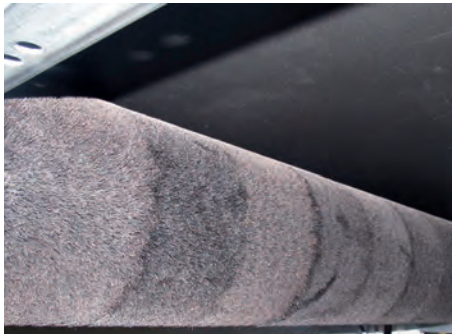
Belt cleaning equipment
